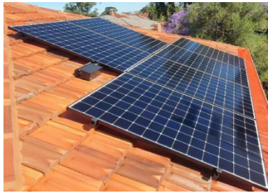
Figure 2. Roof type SunPower Panels
